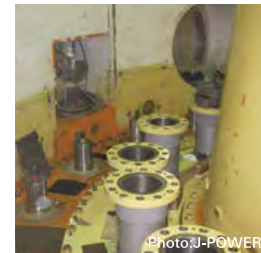
Wicket Gate Control Rod Bushings
