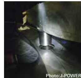
Lower Wicket Gate Bushings
