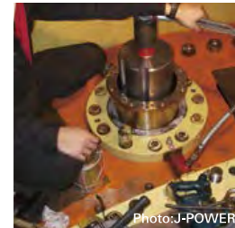
Upper Wicket Gate Bushings
