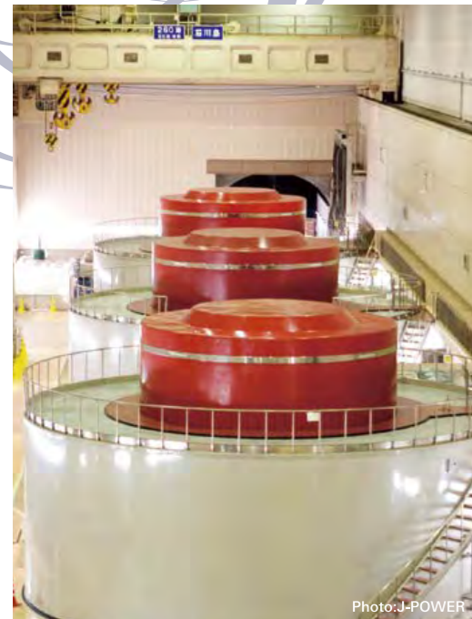
Okutadami Power Station
